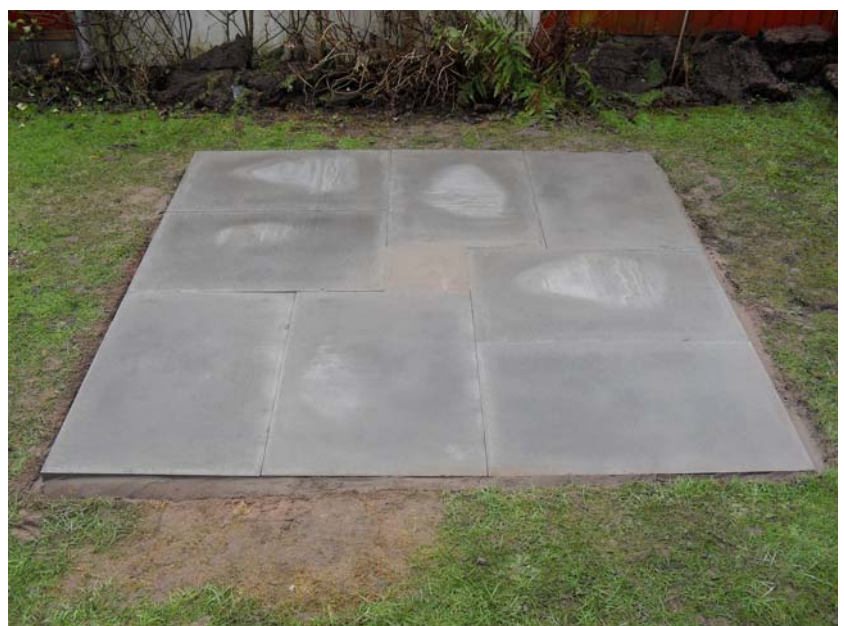
Above: This 7x7 paving slab base would be ideal for a 6x6 summerhouse
